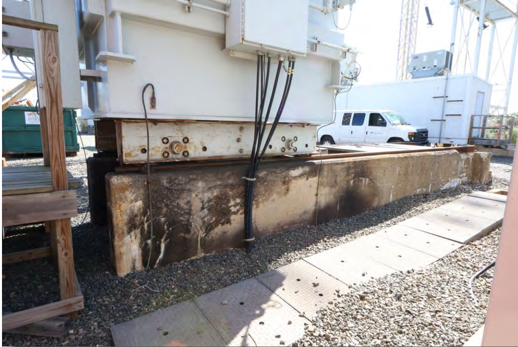
Plate 4.23: Detail of modern transformer mounted on a rail system and concrete pad within Substation 41.
