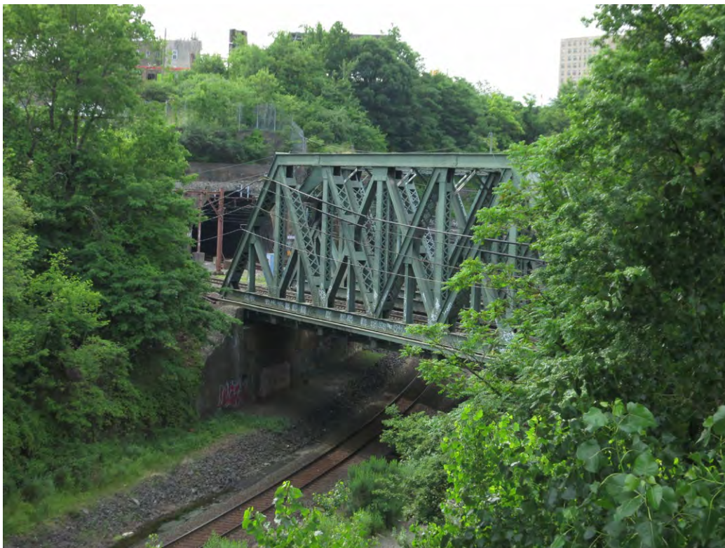
Plate 4.34: View of the West-End Through Truss Bridges and entrance to the Erie Railroad Bergen Hill Tunnel within the Erie Railroad Main Line Historic District, City of Jersey City.
