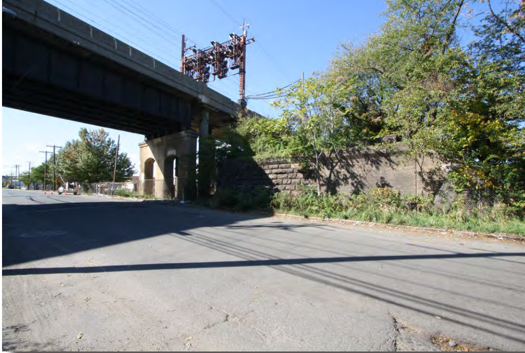
Plate 4.9: General view of the east approach to the Lower Hack Draw Bridge along the Old Main DL&WRR Historic District right-of-way where it crosses Duffield Avenue, City of Jersey City.
