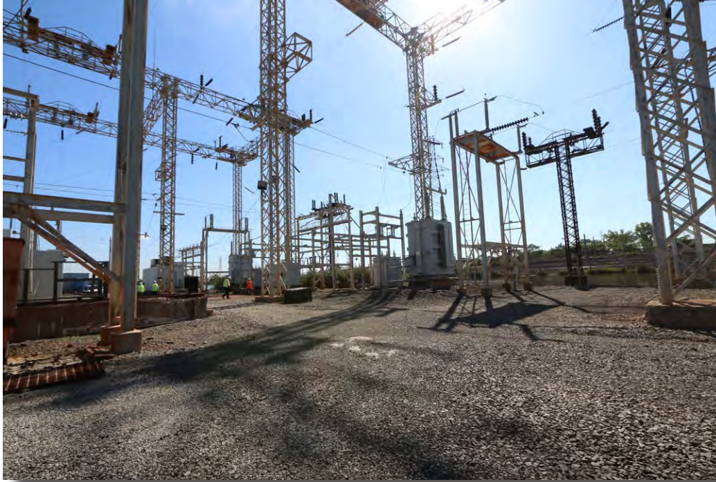
Plate 4.21: Overview of Substation 41, with the Pennsylvania Railroad New York to Philadelphia Historic District right-of-way visible in the background.
