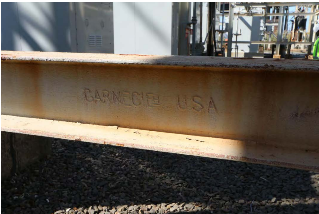
Plate 4.26: Detail of circa 1930 "CARNEGIE H USA" I-beam within the steel structural system, located immediately west of the extant transformers.
