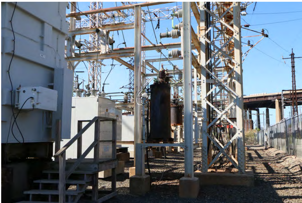
Plate 4.24: View of steel support structures and two extant late 1920s transformers.
