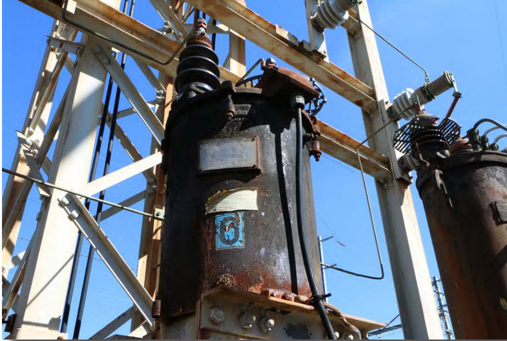
Plate 4.25: Detail of General Electric Company transformer with part of the American Brown Boven Company transformer at right.
