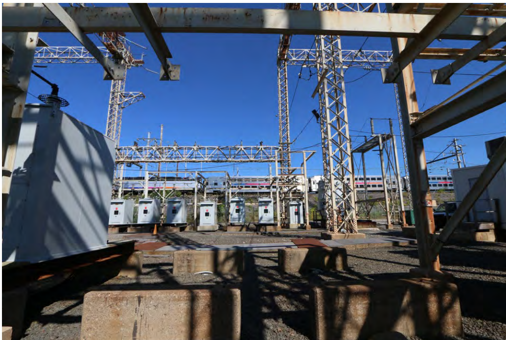
Plate 4.22: View of steel support structures, concrete pads, and transformers within Substation 41, with the Pennsylvania Railroad New York to Philadelphia Historic District right-of-way visible in the background.
