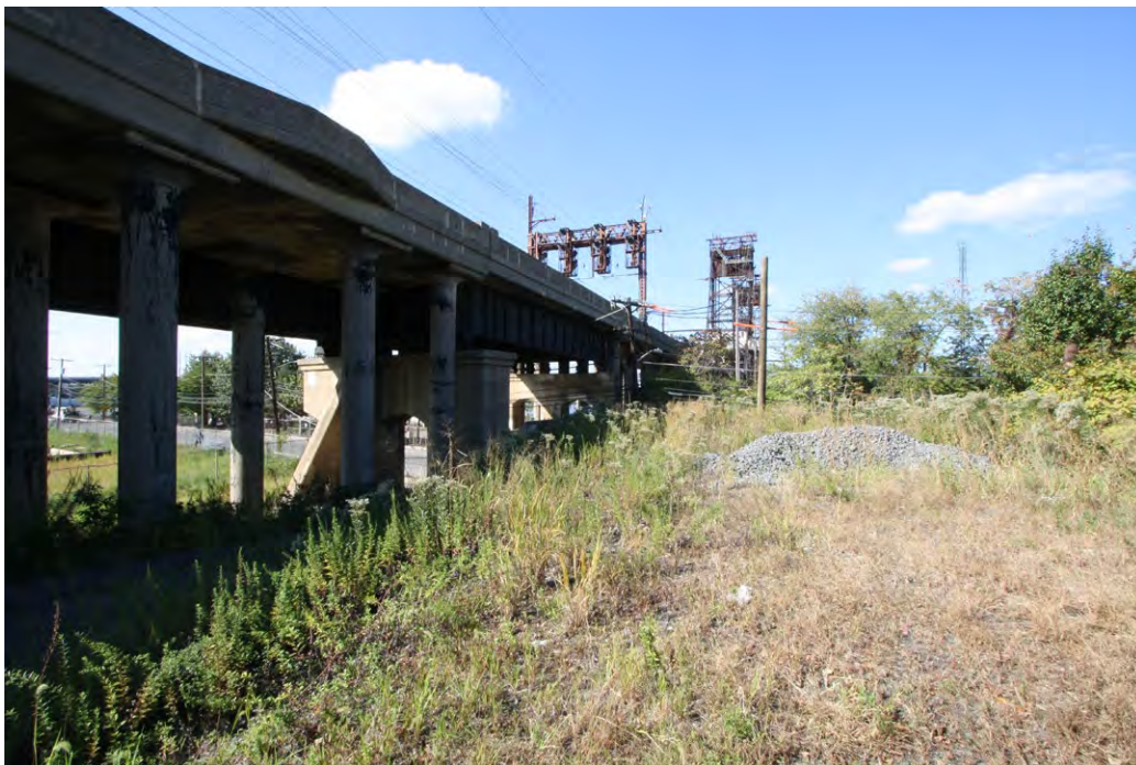
Plate 4.4: Overview of the Old Main DL&WRR Historic District, City of Jersey City.
