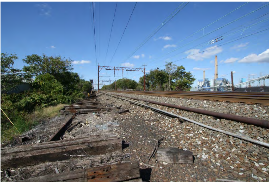
Plate 4.6: Overview of the Old Main DL&WRR Historic District, City of Jersey City.
