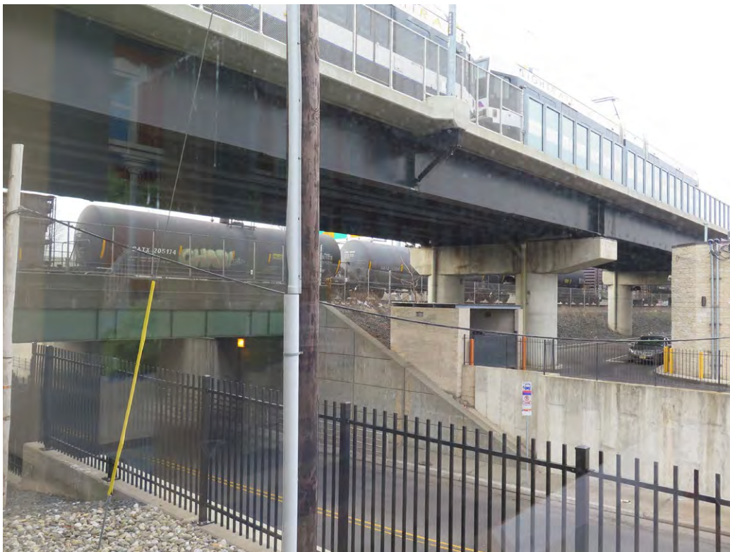
Plate 5.6: Overview of the ground surface at Eighth Street Station, the southern terminus of the HBLR, City of Bayonne.
